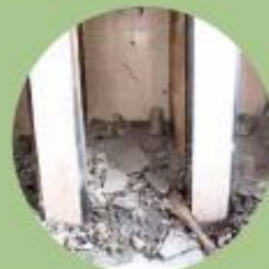
Lack of maintenance, leakage in pipe drainage systems, foul smell.
