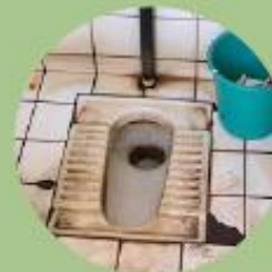
Lack of cleanliness, various kinds of hygiene issues, due to poor maintenance.
