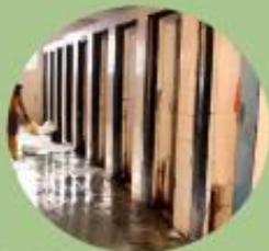
Water on floors can lead to slippery action, broken doors, lack of security.
