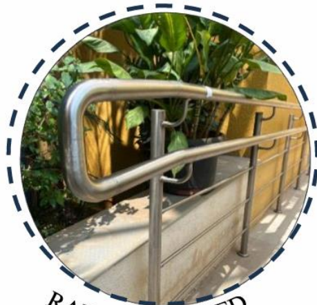
RAILING TURNED DOWNWARDS
