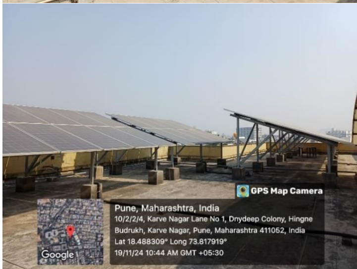
Rooftop solar plant at BNCA
