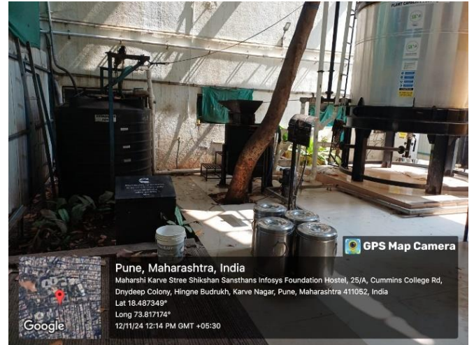
Biogas plant on the MKSSS campus
