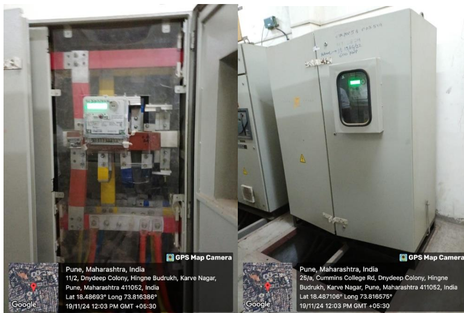
Central net meter on the MKSSS CAMPUS
