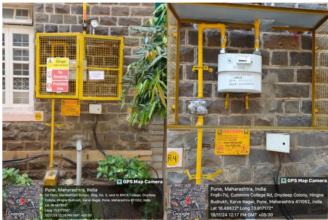
Maharashtra Natural Gas meter for the BNCA canteen on the MKSSS campus
