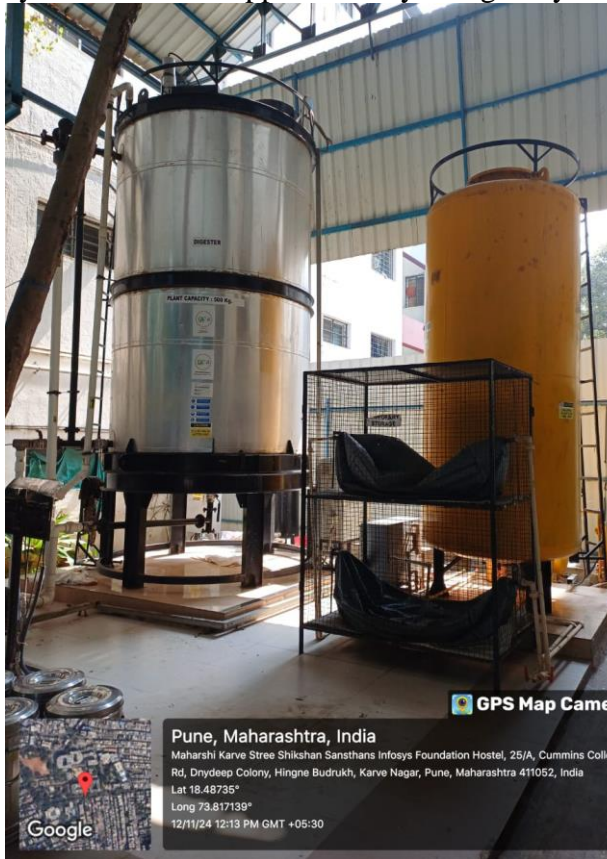
Biogas plant on the MKSSS campus
