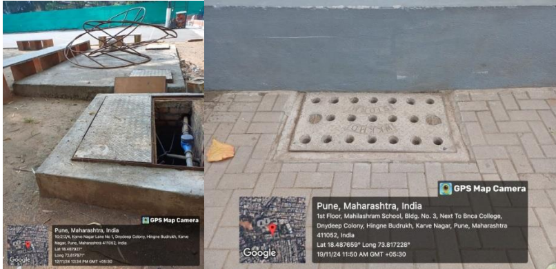
Recharge borewell and stormwater collection system
